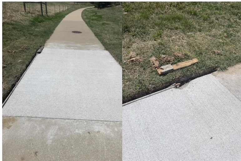
T3 COMPLETE BUT DAMAGED
